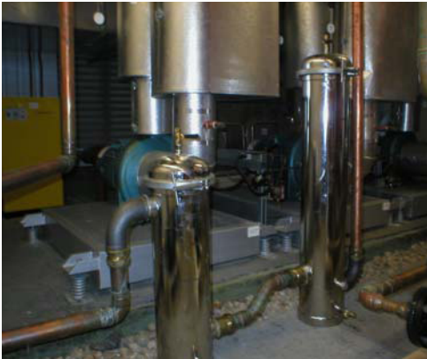
Typical installations with magnetic prefilter upstream of disposable cartridge filter
