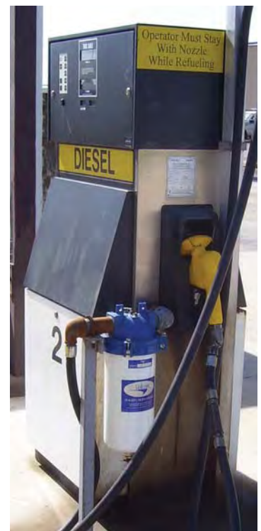
VF-61 connected to a diesel fuel dispenser
